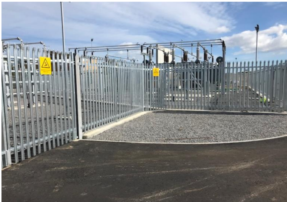
Typical substation complex fencing
