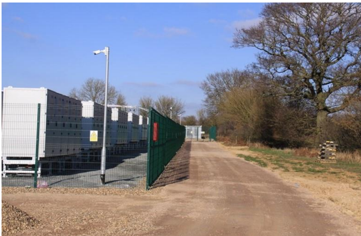
LLPS 17 fencing at BESS site
