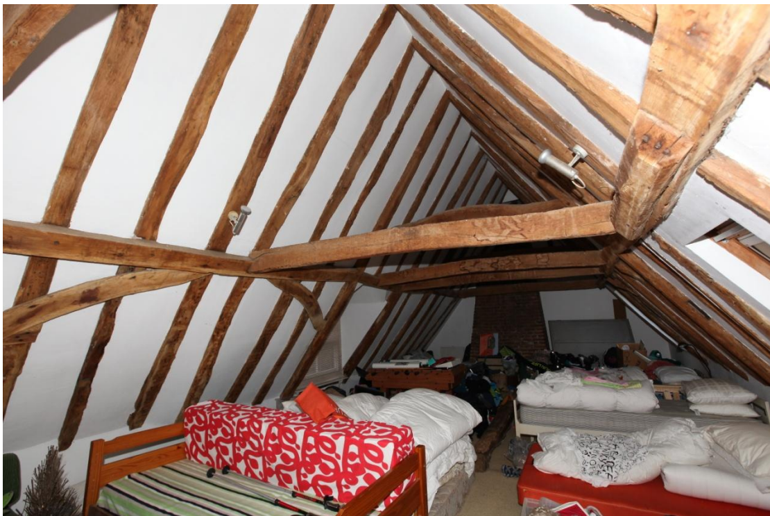
Illus. 38. The roof structure of the 16 th century range looking towards the chimney at its south-eastern gable. The hip rafters beyond this chimney are re-used, narrow-sectioned timbers that are likely to date only from the late-19 th century refurbishment. The linear butt-purlin roof was fully wind-braced, although only a small number of these curved timbers survive. There is no evidence of original dormer windows and the rafters may have been exposed to the first-floor chambers initially (as in the earlier parlour wing).
