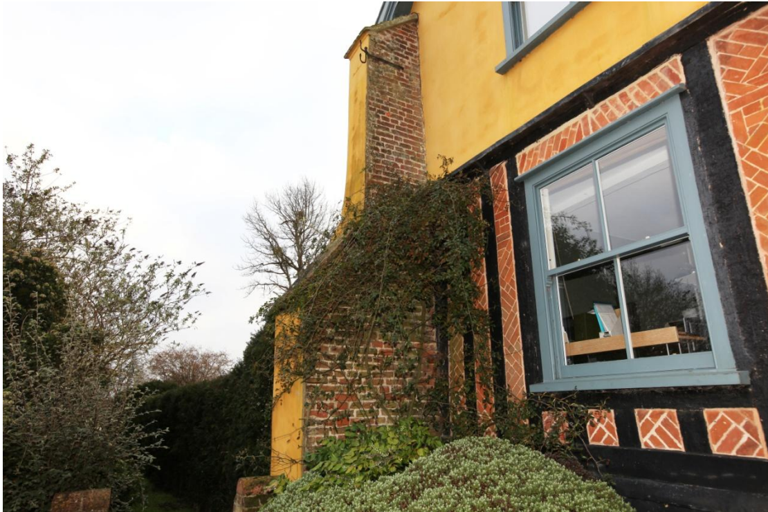
Illus. 3. The buttness of 17 th century brickwork to the left of the facade, which is matched by another to the rear (illustration 5). The bricks are broken at the left-hand edge, indicating its present shape is secondary, and these features probably represent the remains of a large brick wing that projected to front and rear.
