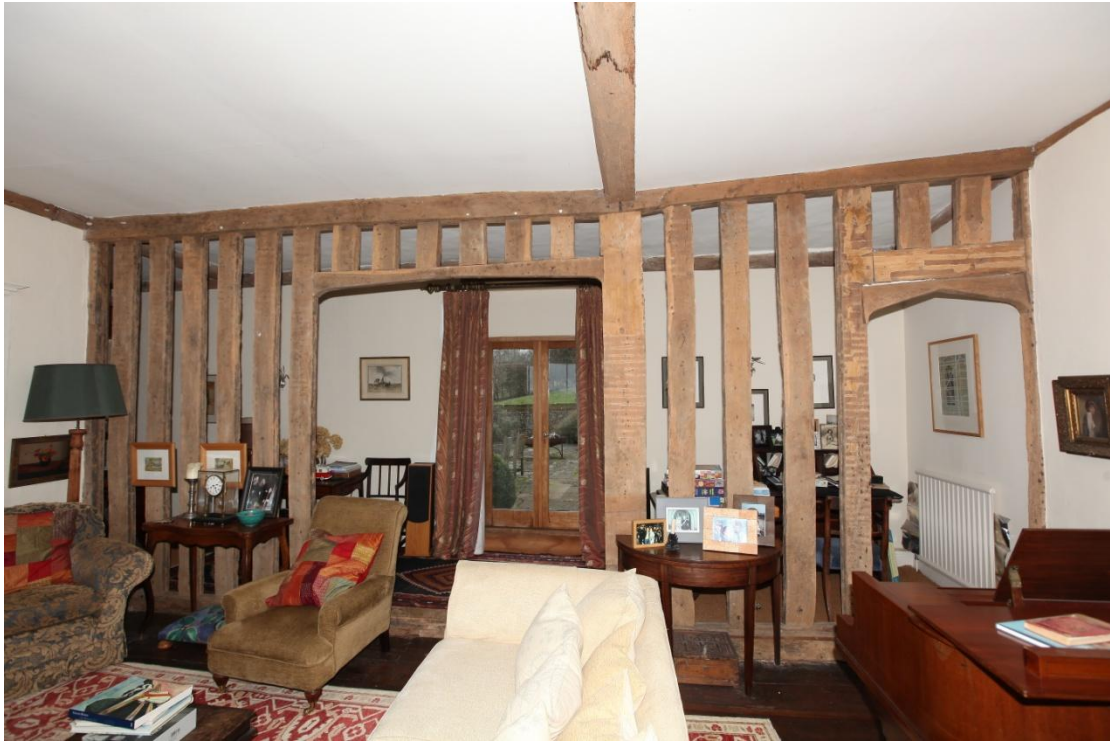
Illus. 25. The closely-spaced studs of the partition between the present sitting room and the jettied 'rear' gallery. The narrow doorway of 0.9 m or 3 ft to the right is an original feature, although its arch cuts its jambs and was inserted after a narrower original door was widened. The wide arch on the left is also a later insertion and there is no evidence of either an original door or window in this bay.
