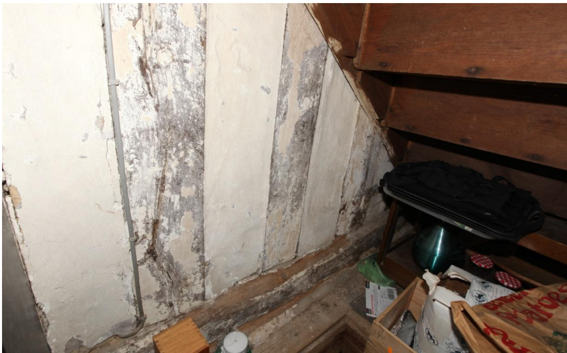
Illus. 10. A detail of the parlour wing's external studs exposed on the cellar steps with the pine boards of the 19 th century main staircase on the right. These timbers are soot-encrusted beneath their later whitewash and evidently faced an open hall on the site of the 16 th century galleried range. The cellar is a small 17 th or 18 th century insertion.
