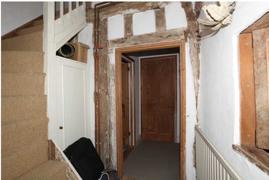
Illus. 14. The upper storey of the parlour cross-wing showing the present attic staircase that still occupies the same narrow bay as the 15 th century main stair (looking north-east towards the sub-divided front parlour chamber with the internal hatch window in illustration 12 on the right). The timbers of the existing door are unpegged insertions.
