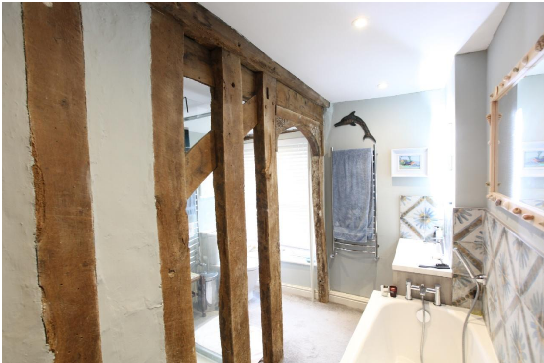
Illus. 16. The rear wall of the front parlour chamber showing the arched door in its north-western corner that opens into the narrow stair bay. This two-bay room was spanned by the tie-beam and crown-post in illustration 18 but its original fabric is currently hidden elsewhere. Much of the plaster in the house may preserve early decorative surfaces such as 16 th and 17 th century wall paintings.
