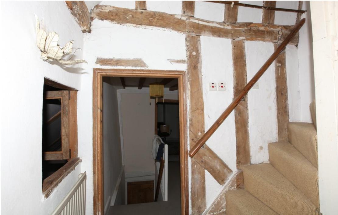
Illus. 15. The inserted first-floor door from the narrow stair bay of the parlour wing to the rear parlour chamber, with the internal hatch in illustration 12 on the left. The doorway cuts an original wall brace as the original stair rose from the ground beneath to the arched door against the north-western side-wall in illustration 16. The upper storey would have been open to its rafters initially, with no need for an attic stair.
