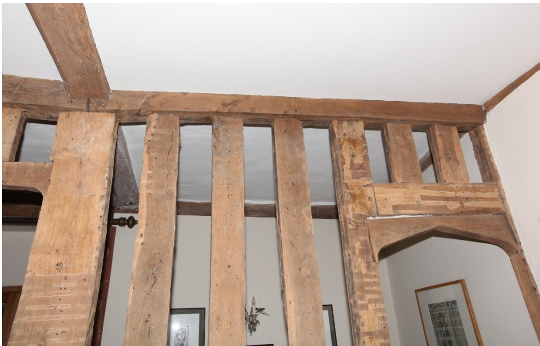
Illus. 26. A detail of the partition in illustration 25. The three studs between the post on the left and the door jamb are later nailed insertions that block a wide former aperture respected by a sharp edge to the binding joist at top left. The door jamb is grooved for brick infill like the other original studs and suggests a chimney once occupied this position, backing onto a cross-passage as often seen in early-16 th century houses.
