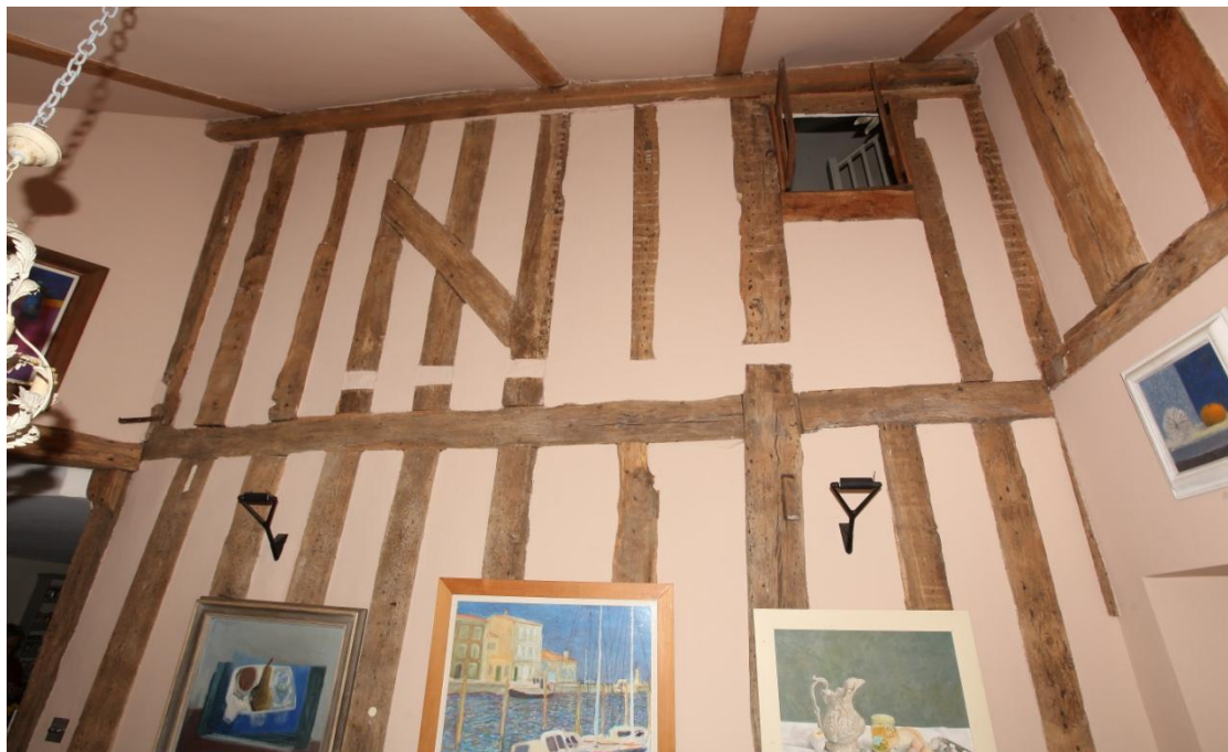
Illus. 12. The external wall of the parlour wing in illustration 11 showing the narrow stair bay on the right. The studs beneath the mid-rail of this bay are later insertions that block a stair door in the rear corner of the missing open hall. Two mortices in the adjoining storey post secured either the latter's back wall or a corner outshot and pegs for an external window sill with moulded mullions indicated by rectangular mortices can be seen to its left. Pegs for a matching first-floor window sill are visible above.
