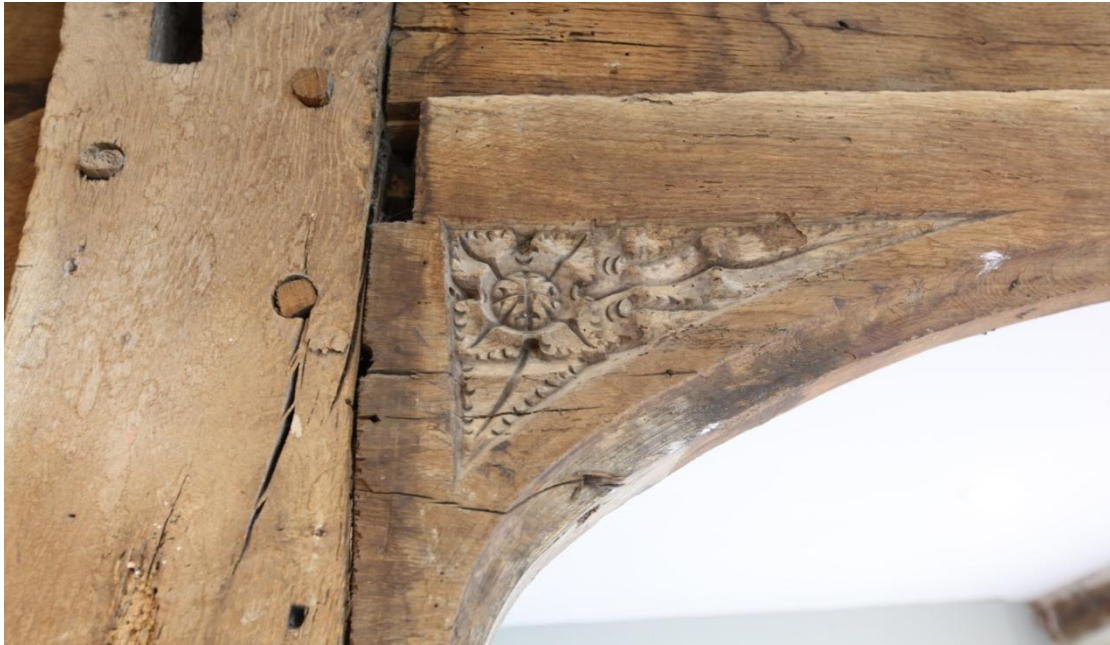
Illus. 17. A detail of a finely carved foliate spandrel to the arched door head in illustration 16. Its counterpart on the right differs slightly. This arch does not fit its current position and is secured by new oak pegs. Its hollow chamfer matches that of the opposite internal edges of its jambs and the timber has been turned around so the carving can be seen from the parlour chamber instead of the stair landing from which it would have been approached initially. A second doorway would have opened from the same landing into the rear parlour chamber.
