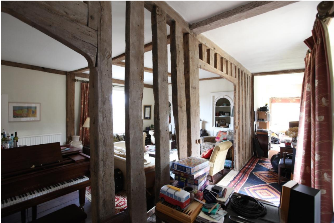
Illus. 29. The gallery from the north-west showing the widened original door on the left and the window that replaced the doorway in illustration 28 at its far end to the right.
