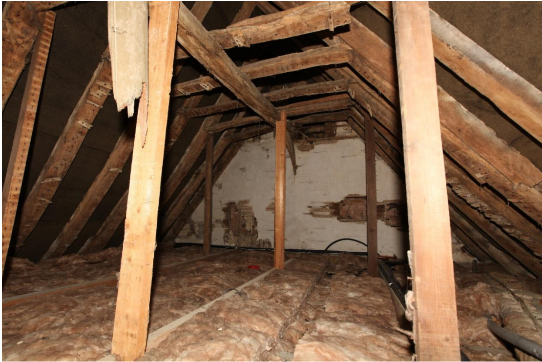
Illus. 21. The roof of the rear parlour chamber showing the probably 17 th century lath-and-plaster of the south-western gable in the rear (as seen from the hole in the partition to the right in illustration 20). The vertical supports are modern. Although the collar purlin is jointed, all five bays of the wing appear to be contemporary.
