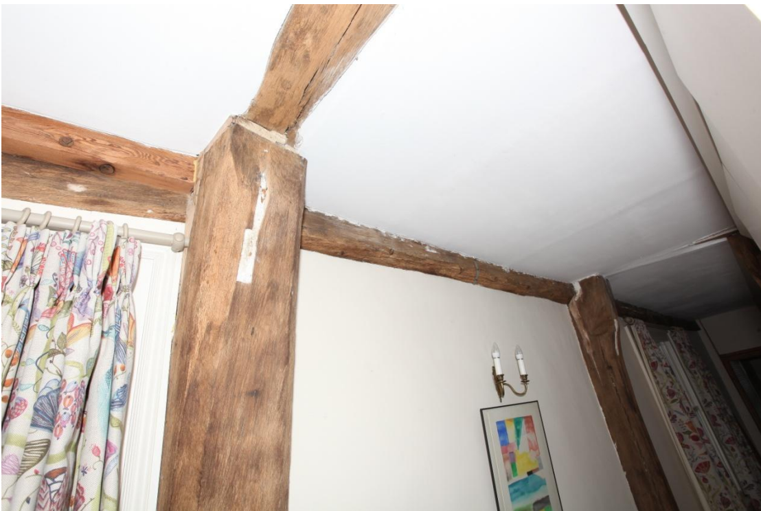
Illus. 36. A detail of the north-eastern roof plate to the right in illustration 32. A stud peg to the right of the jowled storey post indicates the position of a first-floor door immediately above the external door in illustration 2. The post to the right contains a mortice for a door lintel behind the missing apparent chimney, but the unpegged mortice in the post to the left may represent an insertion as there are no stud mortices for a corresponding partition in the tie-beam above.
