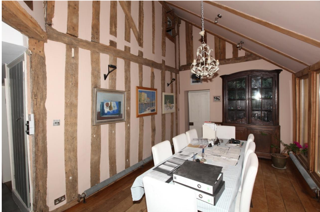
Illus. 11. The south-eastern external wall of the parlour cross-wing seen from its 20 th century lean-to addition. Its junction with the jettied 16 th century range is visible in the rear. The wall of the rear bay on the extreme left has been removed entirely to create an open-plan kitchen/dining room and the internal ceiling joists and wall studs of both rear bays are hidden.
