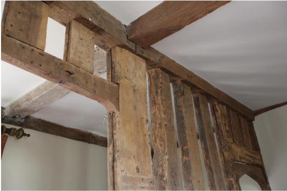
Illus. 27. A detail of the gallery framing showing the V-shaped grooves in the sides of all the original timbers but absent from the three insertions. These grooves were designed to secure infill panels of brick rather than wattle-and-daub, while the insertions contain the typical holes and notches for horizontal wattle staves.
