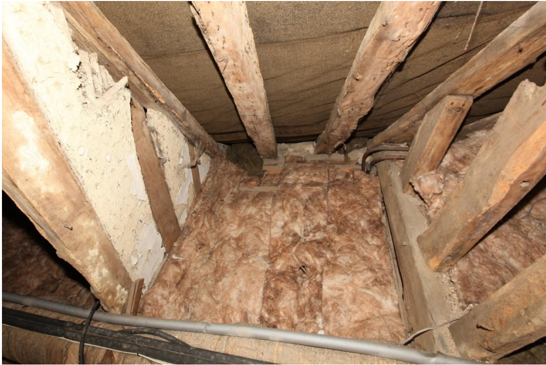
Illus. 19. The narrow stair bay, as seen from the roof, with the studs of the front parlour chamber on the right and those of the central chamber retaining their original wattle-and-daub on the left. This area lay above the stair landing which now forms a shower room entered by the arched door in illustration 16.
