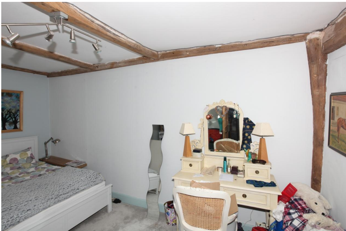
Illus. 34. The bedroom above the north-western bay of the ground-floor sitting room, looking south-east towards the wall above its open truss. The tie-beam contains pegs for a solid wall above the jetty and ground-floor gallery to the right of the central ceiling joist, but both its chamfer and pegs then terminate where the timber was adjoined by a missing chimney (illus. 35). At least some of the exposed joists appear to be insertions.
